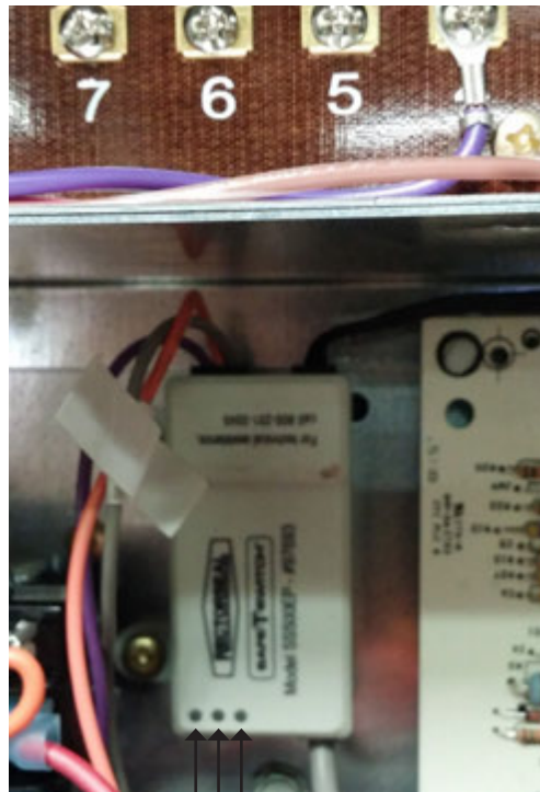
FIGURE 36 Outdoor Condensate Control
