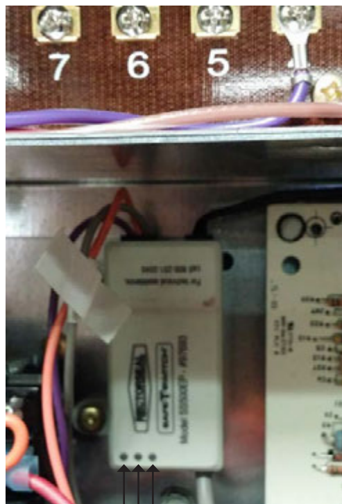
FIGURE 19 Outdoor Condensate Control
