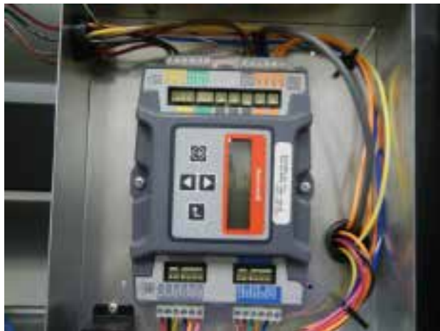
FIGURE 9 Wire Harness to JADE™ Controller
