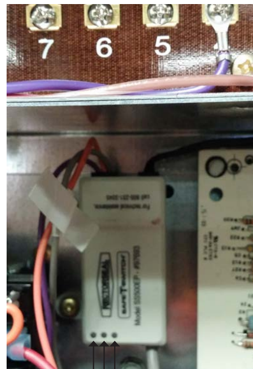
FIGURE 20 Outdoor Condensate Control
