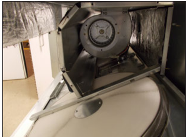
FIGURE 33 Upper Blower Assembly Over Cassettes
