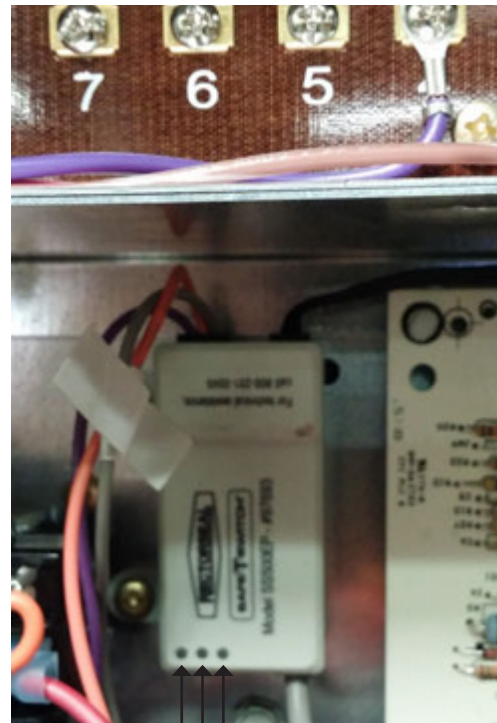
FIGURE 36 Outdoor Condensate Control
