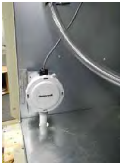
PHOTO #2 OPERATING POSITION
