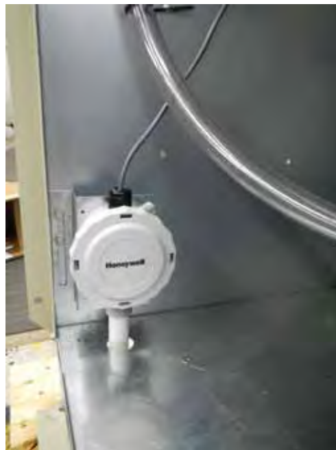
PHOTO #2 OPERATING POSITION
