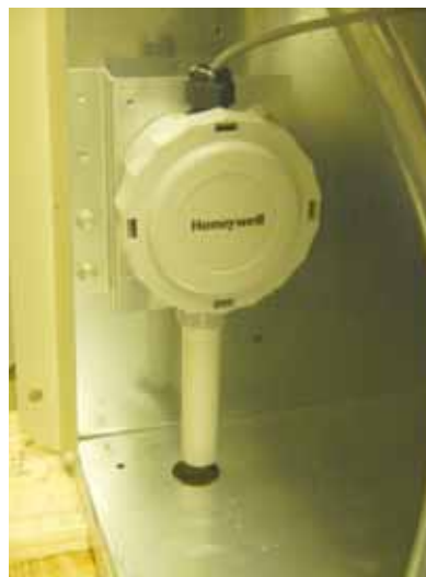
PHOTO #1 OPERATING POSITION
