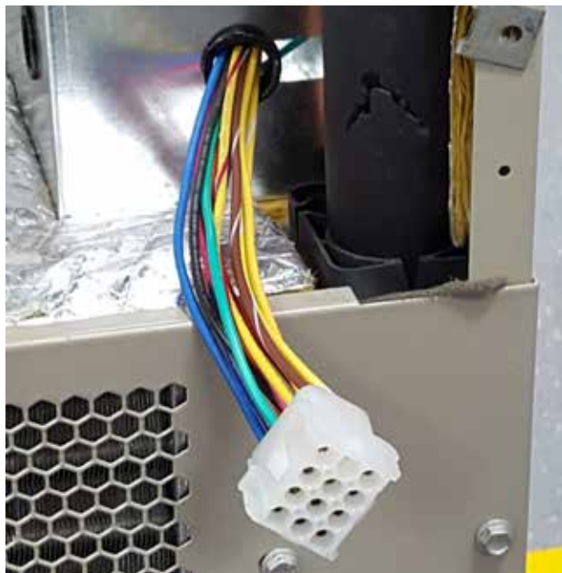
FIGURE 12 Low Voltage Wire Harness Pulled Through Grommet
